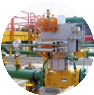
HIPPS with two Mokveld mechanical initiators protecting Shell Tutong metering station in Brunei.
