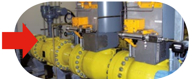
HIPPS prevent over-pressurization by shutting down the source of the high pressure.
